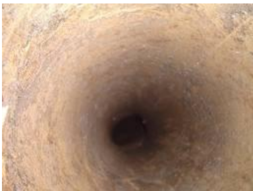
Flue after chimney sweeping
