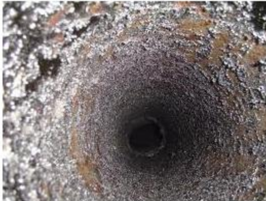
Flue before chimney sweeping
